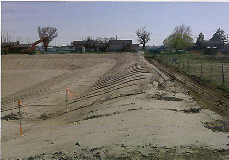
Photo 1. The irrigation reservoir prior to the installation of an EPDM liner. The storage and pressurized system helped balance the area's residential and farm water needs.
